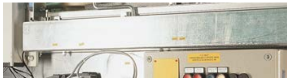
Figure 6-25 Cable installed in cable duct
